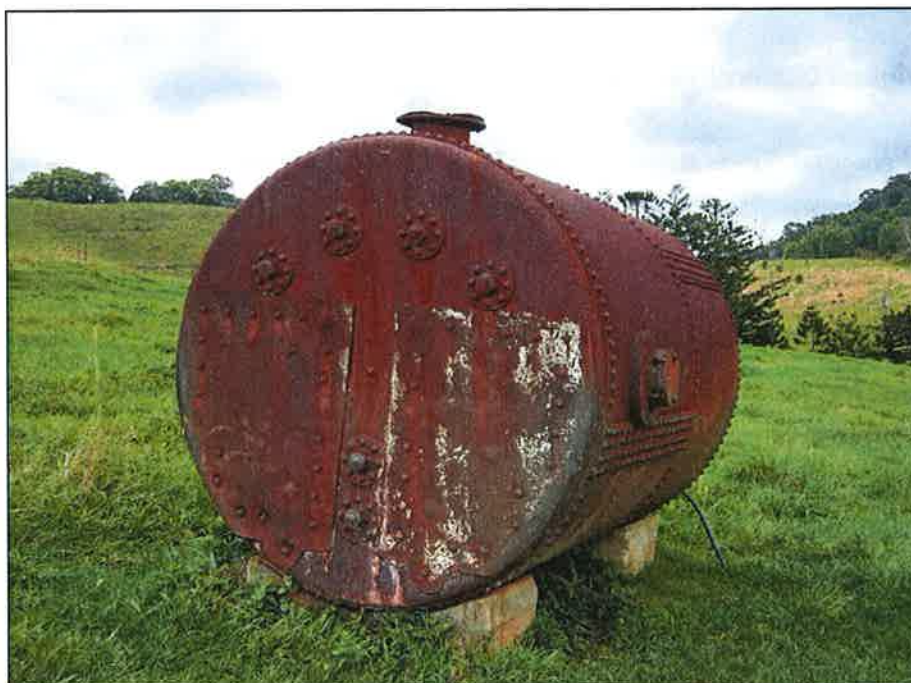
Figure 22: View of Steam Boiler
